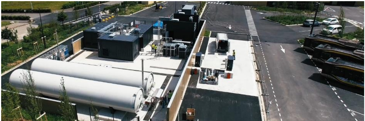
Haut de France, "SMT- AG" project: first zero-carbon hydrogen station for buses in France (200 kg of hydrogen / day, 0.5 MW electrolysis).
