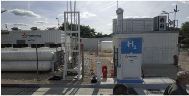
AuxHYGen | Forerunner project for low-carbon mobility concerning heavy-duty transport in France. In 2019 the Artois-Gohelle mixed transport association (SMT AG) ordered a McFilling® station and a Mclyzer® electrolyzer from McPhy to fill six hydrogen buses.
