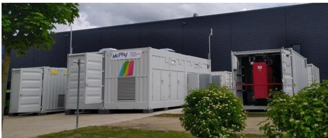
2MW high-power electrolysis McLyzer by McPhy | Apex Energy, Laage, Germany
